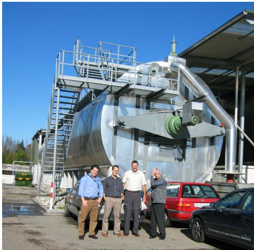
Evergreen Energy Site Visit to KOMPOGAS plant in Switzerland Cylinder in background is the Anaerobic Digester.
