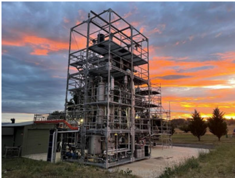
Above: SEATA Pilot Facility - Clean Energy and Carbon Sequestration R&D Centre, Glen Innes NSW (New England REZ).
