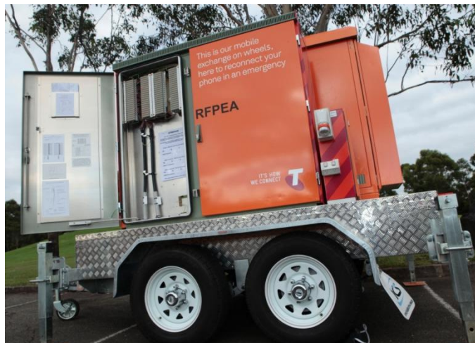
Figure 3: A Mobile Exchange on Wheels (MEOW)
