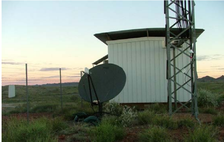
Figure 2: A Satellite Cell on Wheels (SatCOW) at Marble Bar 200Kms S/E of Port Hedland in WA
