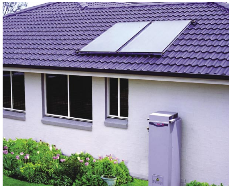
Solar and gas hot water heating
