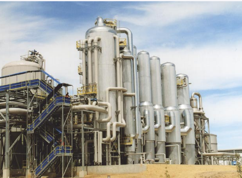
VISY black liquor cogeneration plant
