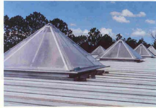
The angular selective skylights.
