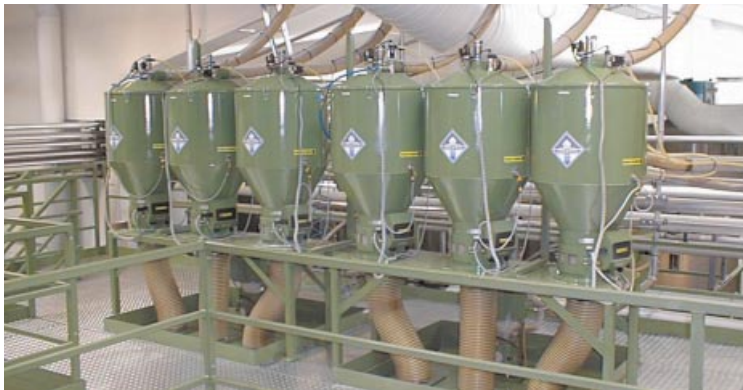
Energy-Efficient Design at Færch Plast A/S has reduced energy consumption by 50%
