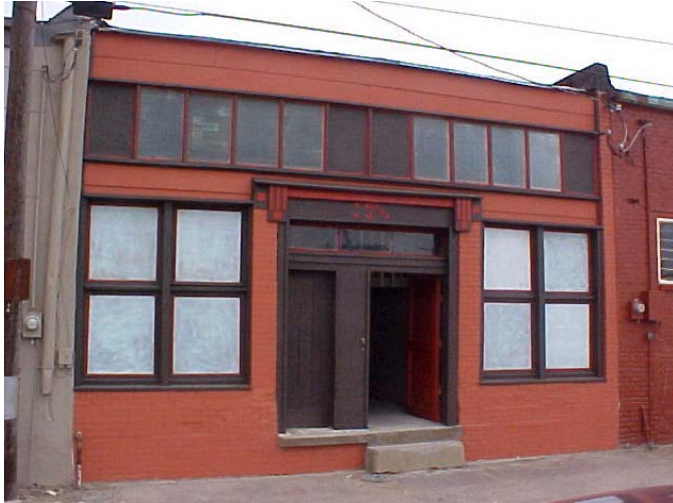
Durant pool hall after restoration as part of the Main Street Program for Durant, Oklahoma. This project was the winner in its category (façade restoration under $10,000) at the Main Street Oklahoma Awards ( http://www.durantmainstreet.org/index.html ).
