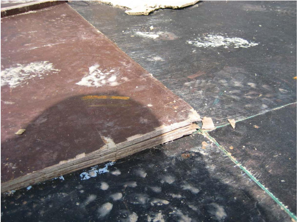
Plate Two – Delaminating formwork plywood in deck
