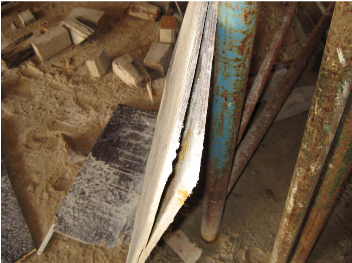
Plate One – Formwork Plywood sheet with severe delamination of the central glue line
